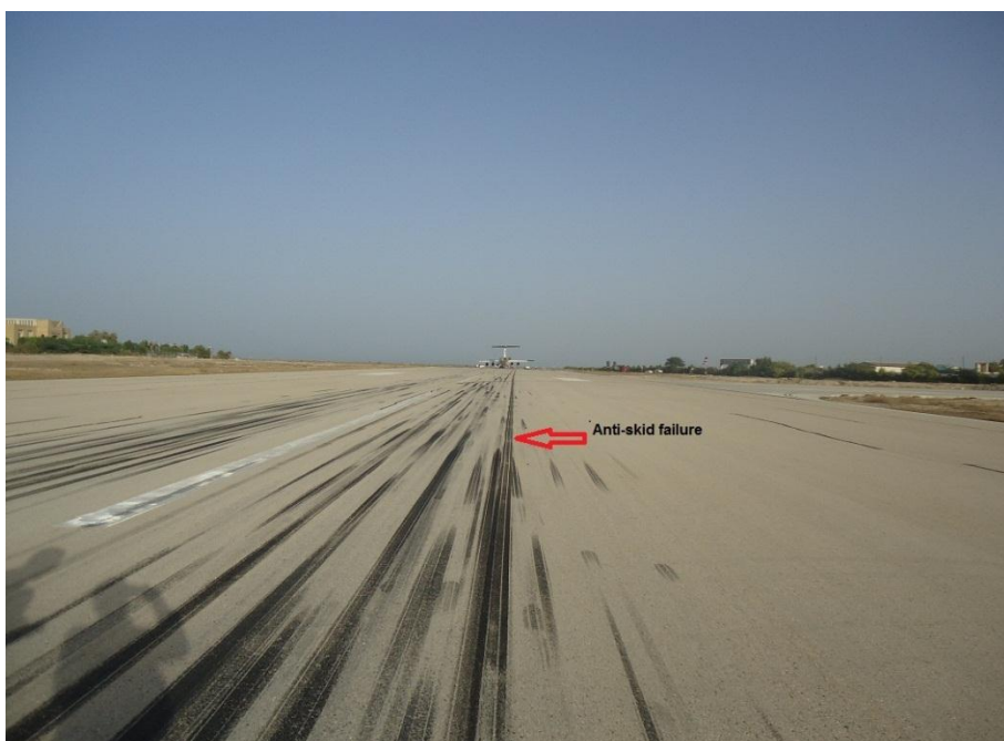
Signs of anti-skid failure
